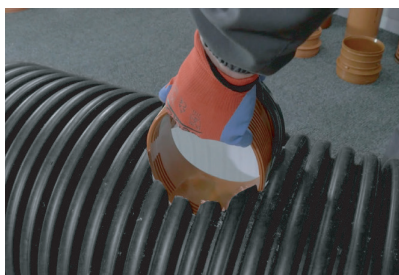
7. Inserting body of sag through pre-prepared opening and setting it in the appropriate position
