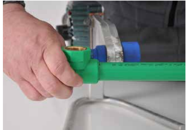
Picture no. 25: Connecting pipes and fittings
