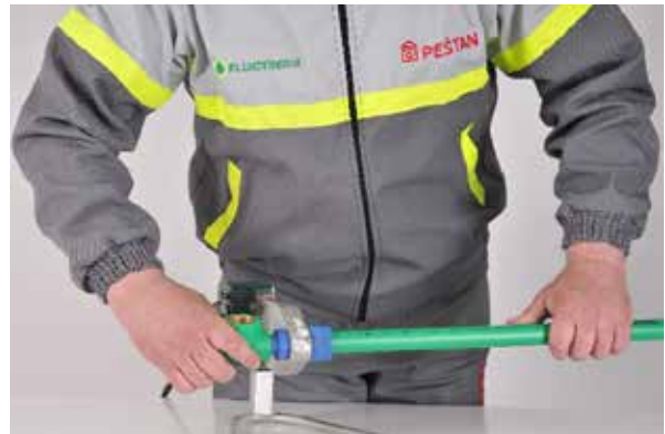
Picture no. 23: Heat pipe and fittings (pay attention to positioning the pipes and fittings on the heating plate)
