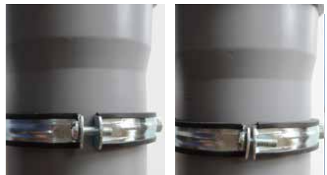
Display of loose and tight clamps on pipes
