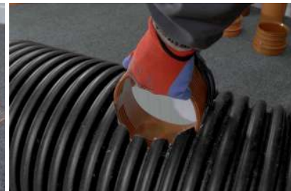
7. Inserting body of sag through pre-prepared opening and setting it in the appropriate position
